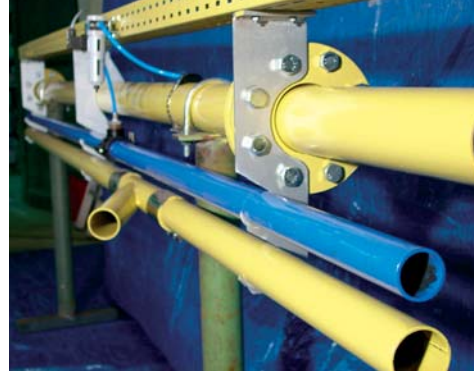
Arrangement of pipes including conveying pipe, compressed air pipe, exhaust air pipe, cable conduit. Compact, space-saving.
